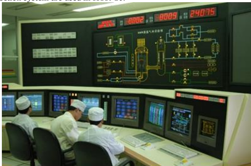
HTR-10 Control room
